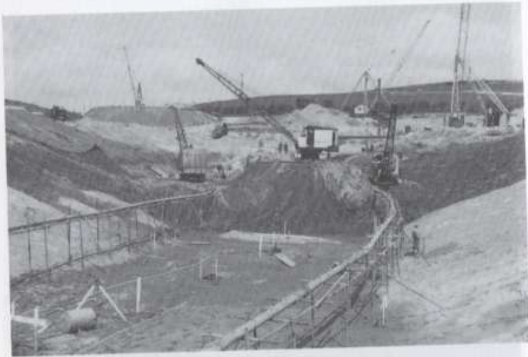
Figure 9.19 Workable conditions, following wellpoint pumping, under which the channel was actually formed (courtesy of Northumbrian Water Limited).
